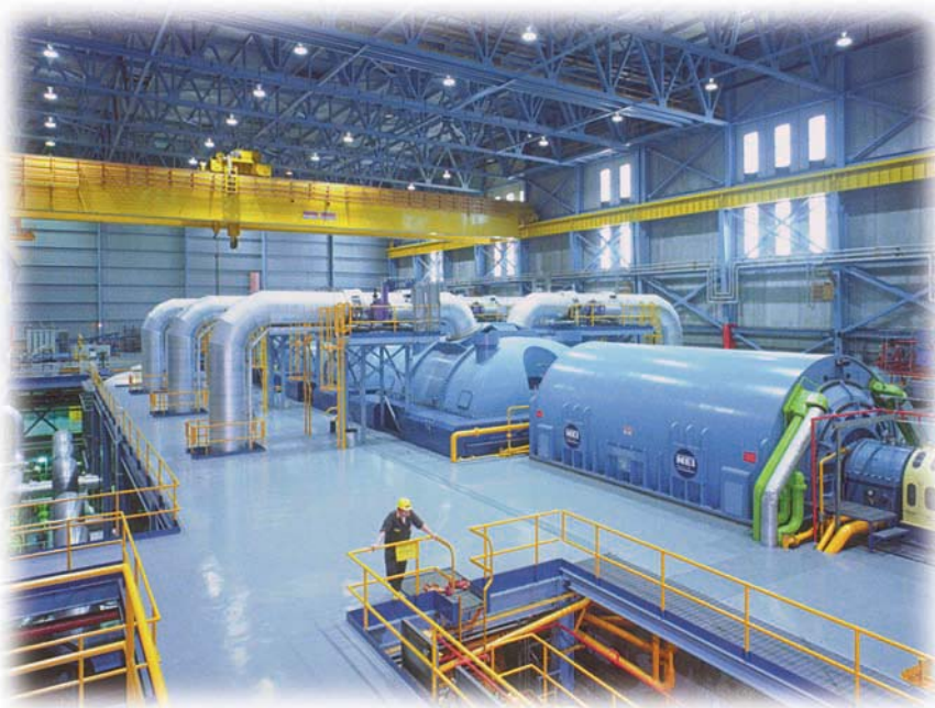
Turbine generators at Point Lepreau nuclear generating station.
